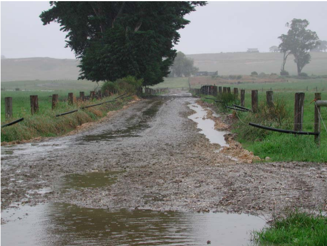
An example of a farm track with inadequate drainage
