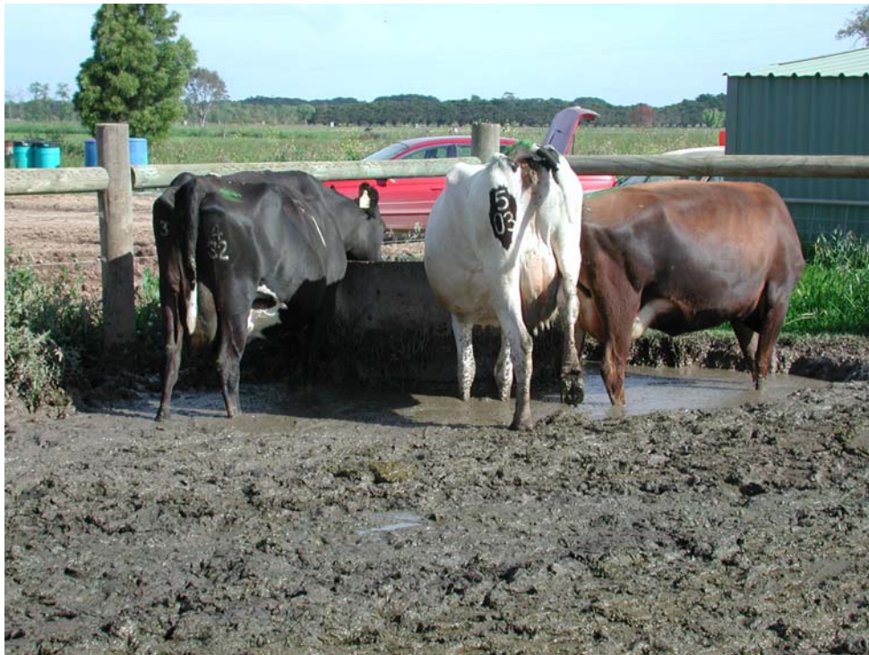
An area around a water trough which is in urgent need of repair. Such wet muddy areas will predispose to lameness.
