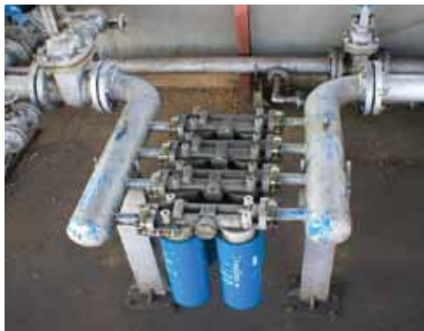
Single-pass Bulk Fuel Filtration System
