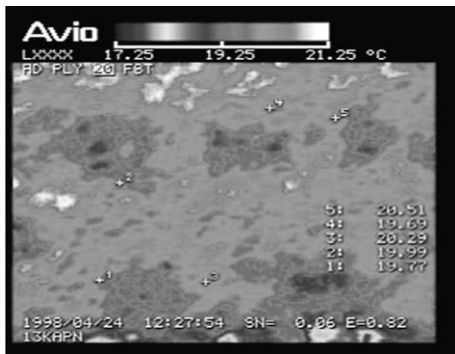
Fig. 12. Thermal image of western facade from the Tobacco Cutting Factory.
