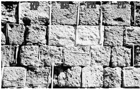
Fig. 6. Consolidated masonry under investigation in the Medieval City of Rhodes (south orientated).
